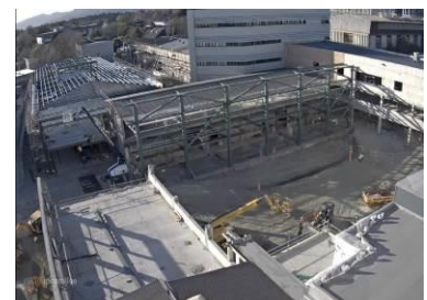
Construction of the engineering core gathers pace with some of the steel frame erected and the roof about to go on the Chemical Engineering wing.
